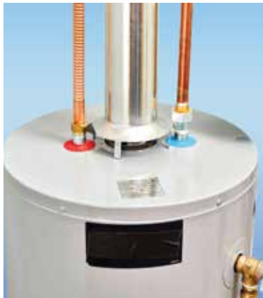
(L) Gas water heater connection
