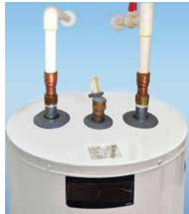
(K) CPVC electric water heater connection
